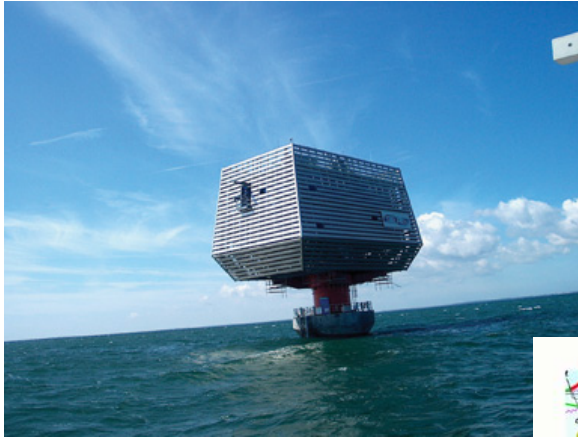
Transformatorstation, Nysted / Rødsans
