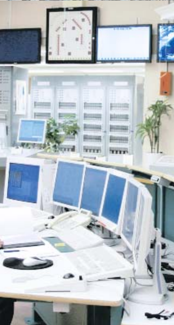
The control room at Forsmark.
