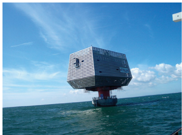
Transformatorstation, Nysted vindkraftspark, DK
