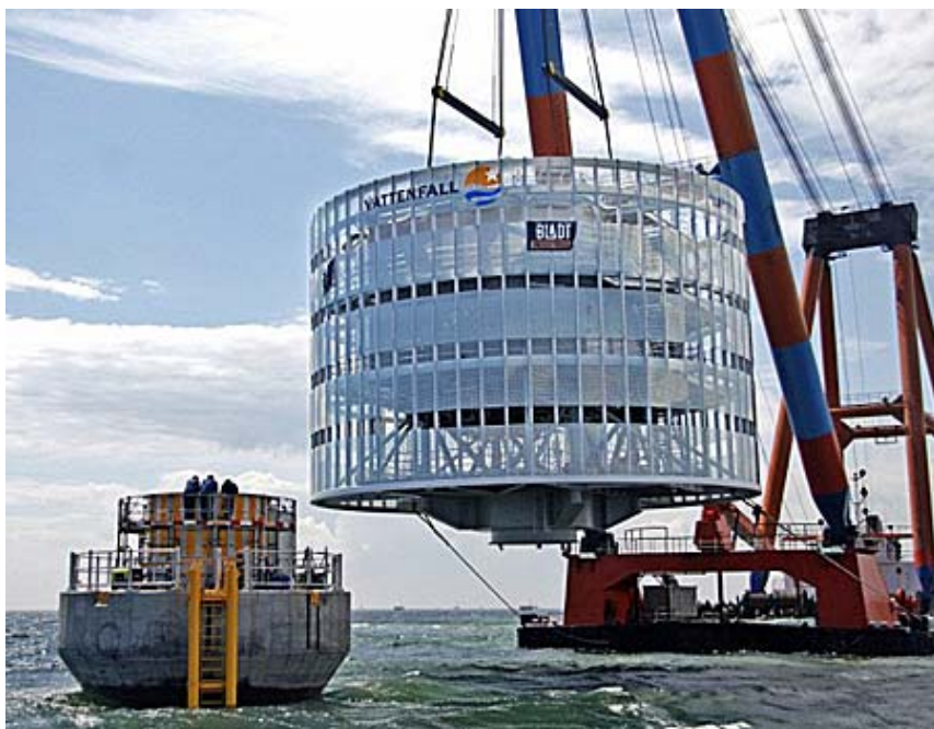
Figure 9: The transformer station was placed on a transition piece of the foundation
