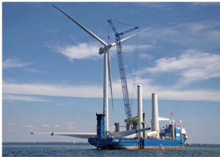
Lillgrund Wind Power Plant 2007-05-04 Installation of a windturbine from M/S See Power.
